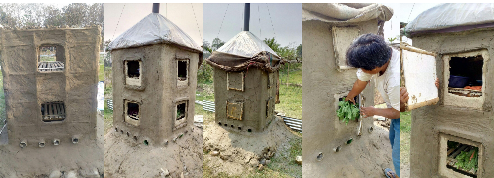
Type B: 1. Cutt the bottom of the bottles for circulation of normal air and also tie up the mouth (inside) with mosquito nets to avoid earth worm, snakes, insects to go inside; 2. Place bamboo scaffolding/ platform (layers will be developed); 3. Openings should be like this and there has to be covers; 4, 5 & 6. Keep vegetables; 7. Locals could understand COLD STORAGE and some data on Temperature.
